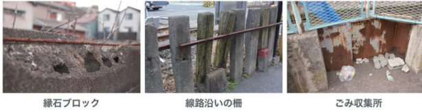
Fig.1 Deterioration of Concrete in Urban Areas
