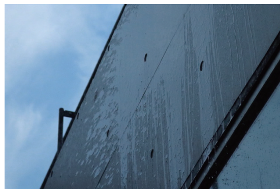
Fig6. Water flow on the surface of exposed concrete
